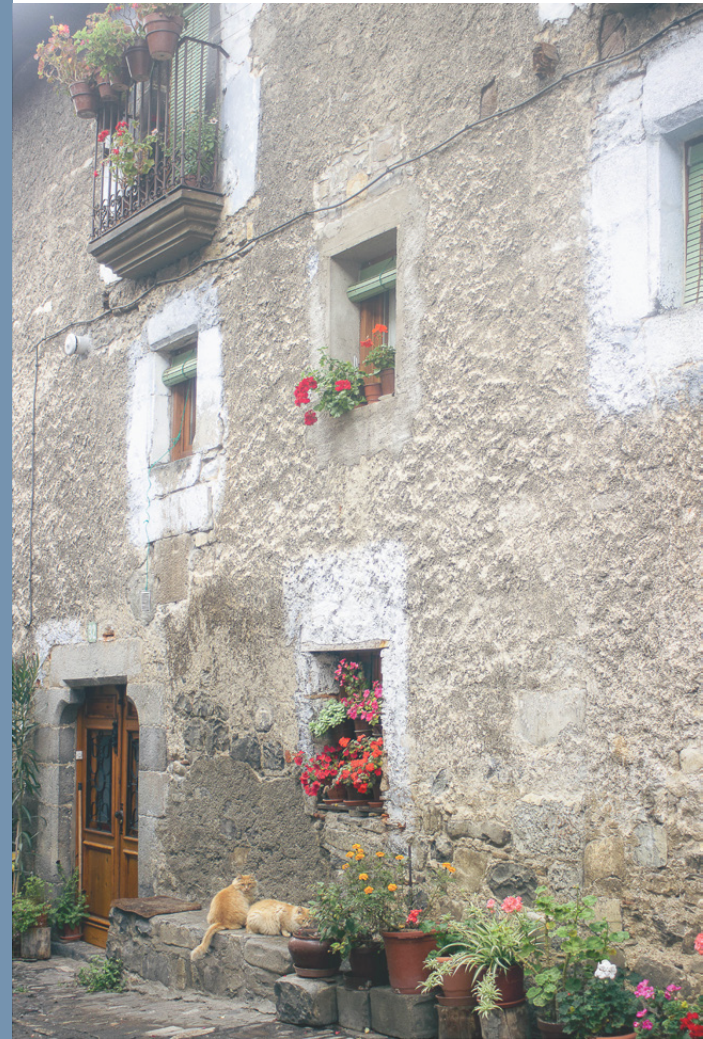
through putting up flowers and painting the wall around the windows, the owner of this house fight against the decay of the building structure
